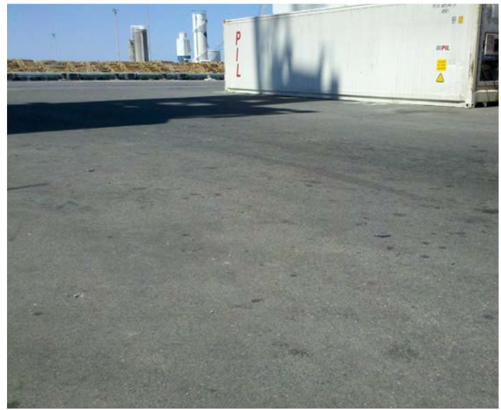
In 2013, three years after placement, freight facility surface shows no visible imperfections
