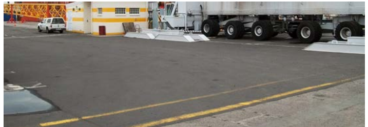
A finished section with HiMA layers at the Port of Napier in December 2010
