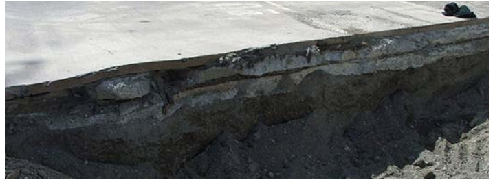
In 2007, the loading area was rutted, failing and in need of replacement
