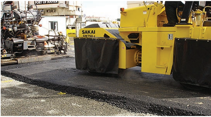
Port of Napier is New Zealand's fourth busiest, with intensive container movements. Initial HiMA lift at Port of Napier was placed in 2010.
